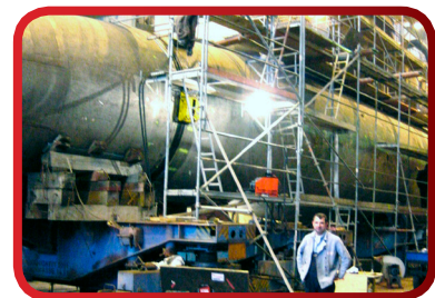
No job is too big for the Trav-L-Cutter, here severing a submarine in dry dock for decommissioning
